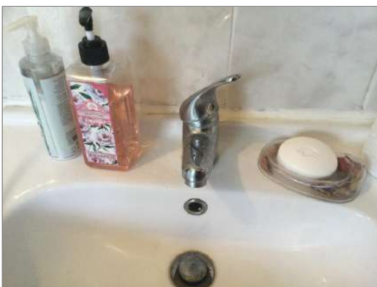
Photo - 124 Cold water was unavailable from the rear shower room tap when operated
