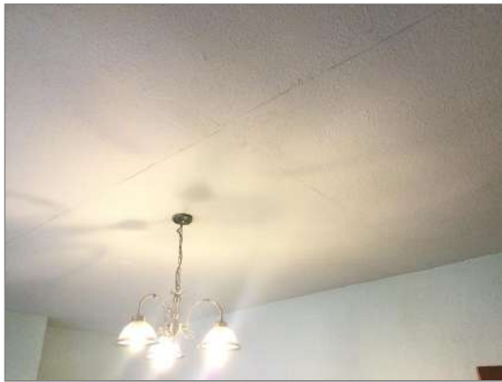
Photo - 77 Cracking was noted to the ceiling in the front bedroom
