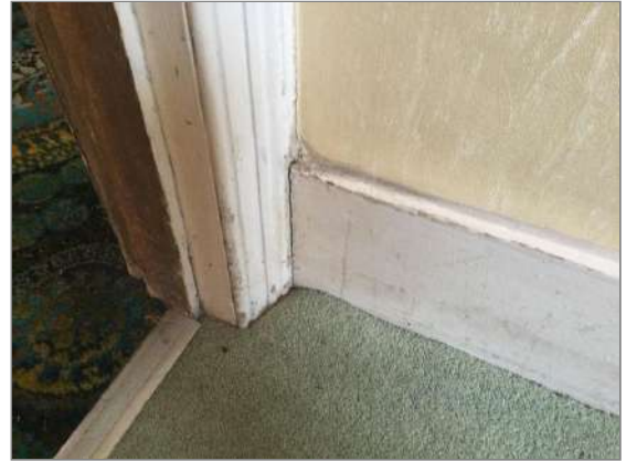
Photo - 116 Example of shrinkage cracking to the skirting boards
