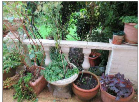
Photo - 145 A crack was noted to the coping stone on the rear garden wall
