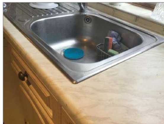
Photo - 112 The sealant was noted to be missing from around the sink
