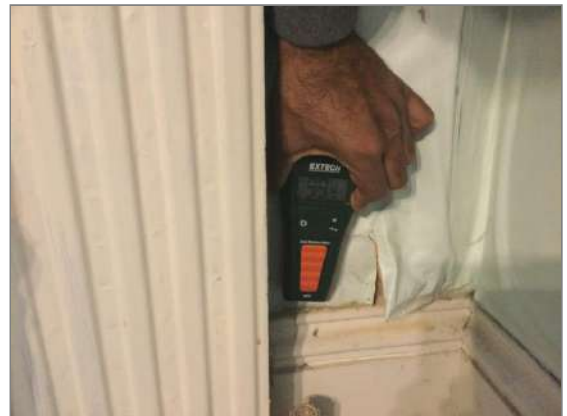
Photo - 90 High moisture meter readings were recorded on the wall in the front bedroom
