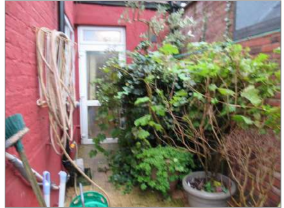
Photo - 149 Overgrown shrubbery was noted to the rear of the property
