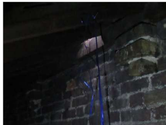
Photo - 67 Gaps were noted to the roof covering
