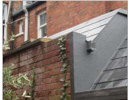
Photo - 151 A coping stone was noted to be removed from the rear right-hand boundary wall
