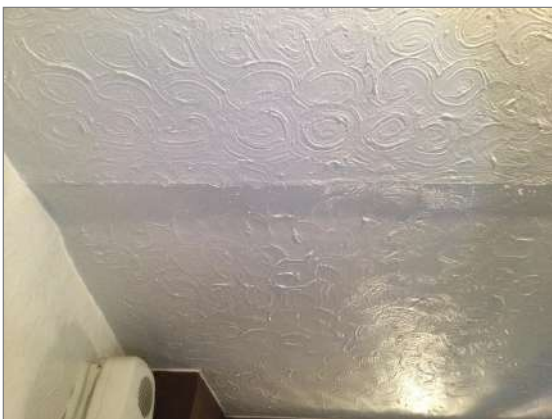
Photo - 75 Cracking was noted to the ceiling in the rear shower room
