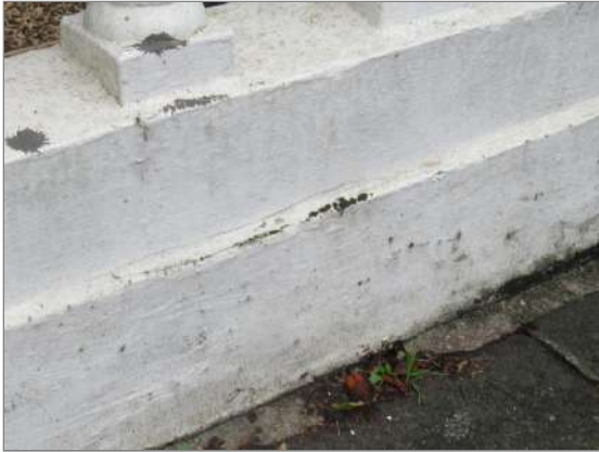
Photo - 136 Cracks were noted to the front boundary wall
