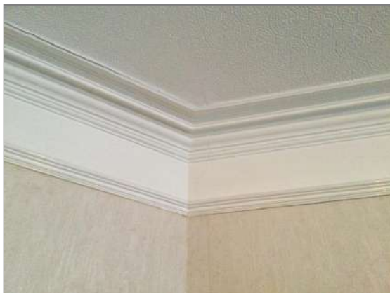
Photo - 69 Hairline cracking was noted to the coving in the front living room
