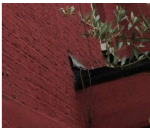
Photo - 22 Gaps were noted to the lead flashing seals of the flat roof
