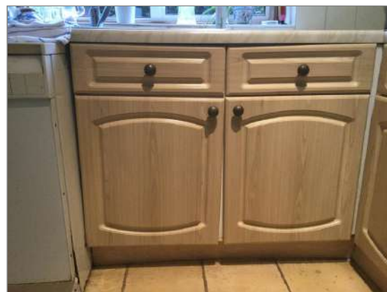
Photo - 110 The cupboard doors were noted to have dropped on their hinges
