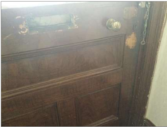
Photo - 51 The front door was noted to be weathered
