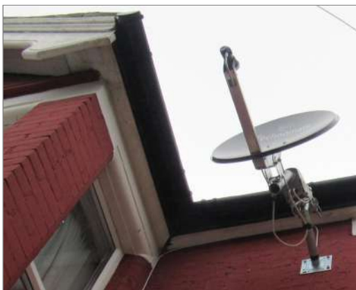
Photo - 59 Weathering was noted to the front elevation soffit and fascia boards
