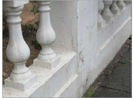
Photo - 137 Cracks were noted to the front boundary wall
