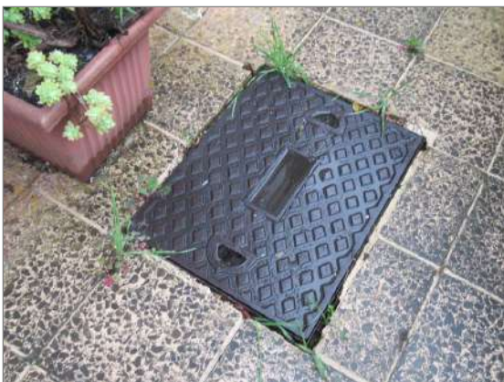
Photo - 140 The manhole cover was noted to rock when traversed on the front elevation
