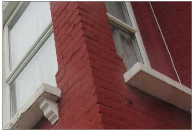
Photo - 36 Damp was noted to the brickwork on the front elevation
