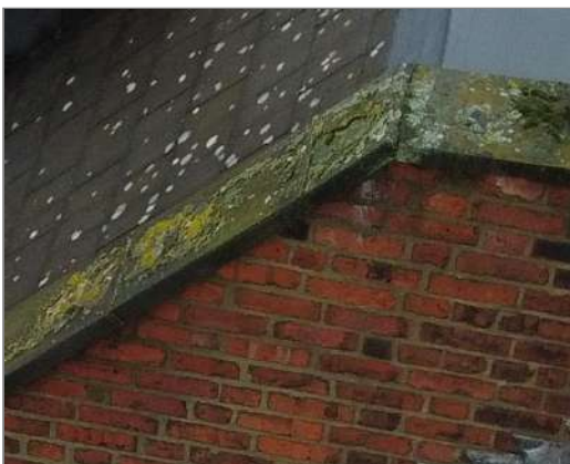
Photo - 18 Moss growth was noted to the joints of the coping stones of the parapet walls
