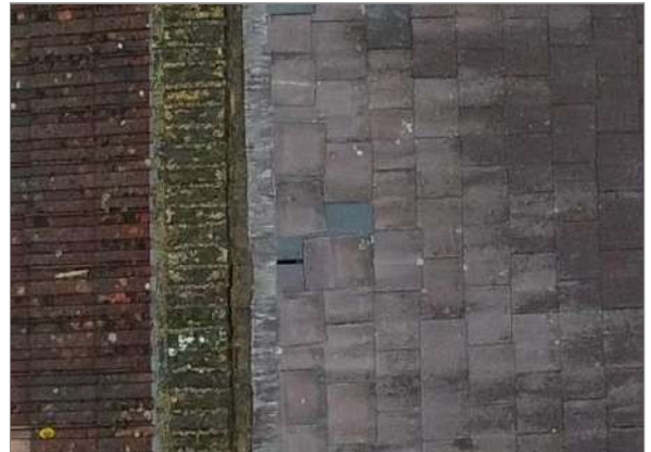
Photo - 17 Gaps were noted between the tiles on the rear elevation main roof
