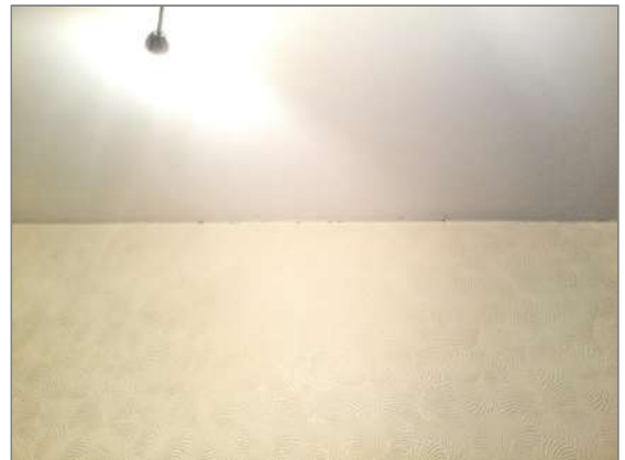
Photo - 74 Perimeter cracking was noted to the ceiling in the rear left shower room
