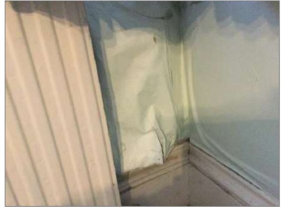
Photo - 82 Damp was noted to the walls in the front bedroom
