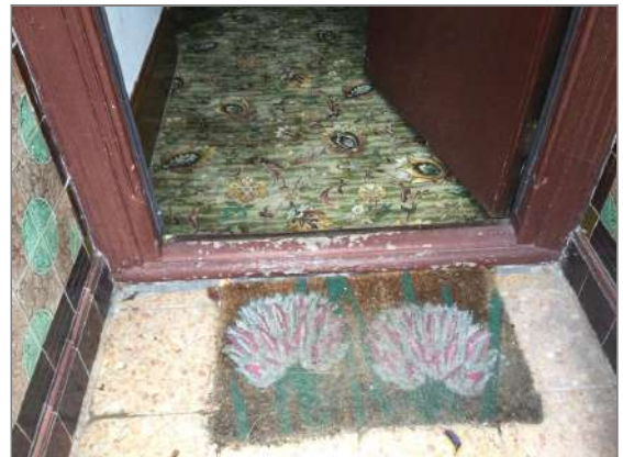
Photo - 50 The front door was noted to be weathered
