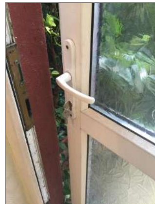
Photo - 54 The rear side door was noted to be defective when operated
