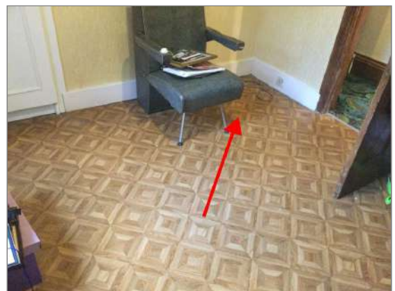
Photo - 102 The flooring in the second left hand bedroom was noted to be sloping
