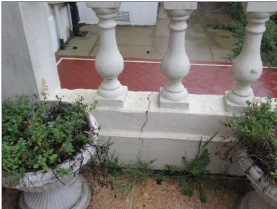
Photo - 138 Cracks were noted to the front right-hand boundary wall
