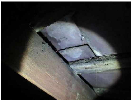
Photo - 64 Damp and mould was noted to the timber roof structure
