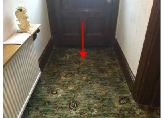
Photo - 98 A dip was noted to the flooring by the front door
