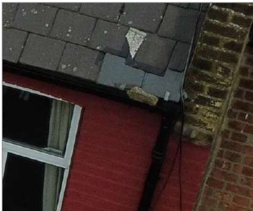
Photo - 27 Items were noted to be blocking the guttering on the rear elevation
