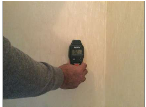
Photo - 94 High moisture meter readings were recorded on the wall in the third left-hand bedroom
