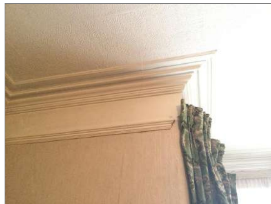
Photo - 70 Hairline cracking was noted to the coving in the front living room
