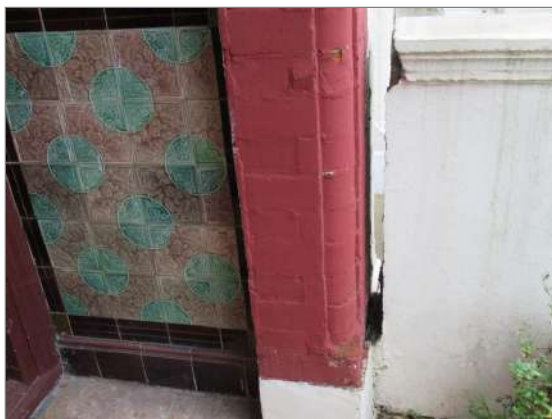
Photo - 33 Damp was noted at the base of the walls on the front elevation
