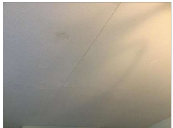
Photo - 76 Cracking was noted to the ceiling in the front bedroom
