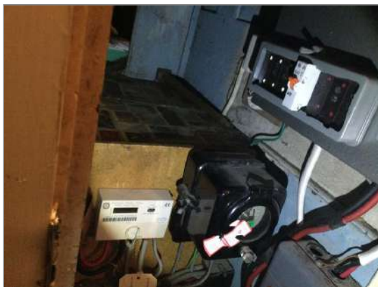
Photo - 127 Electricity meter and consumer unit
