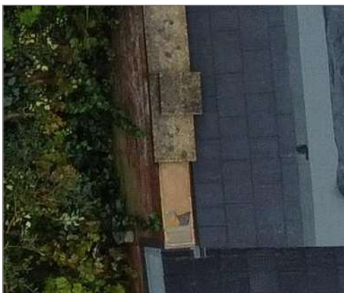
Photo - 152 A coping stone was noted to be removed from the rear right-hand boundary wall
