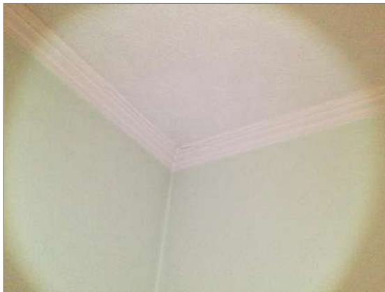
Photo - 79 Hairline cracking was noted to the coving in the first left hand bedroom
