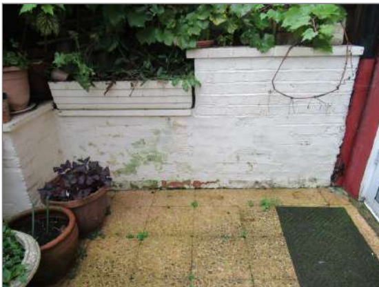
Photo - 144 Damp was noted to the rear right-hand boundary wall
