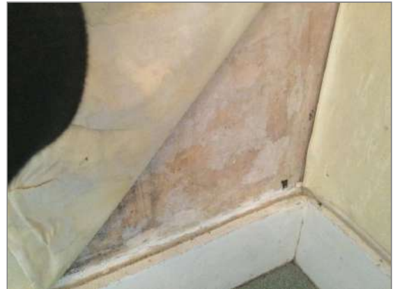
Photo - 84 Damp was noted to the wall in the third left hand bedroom
