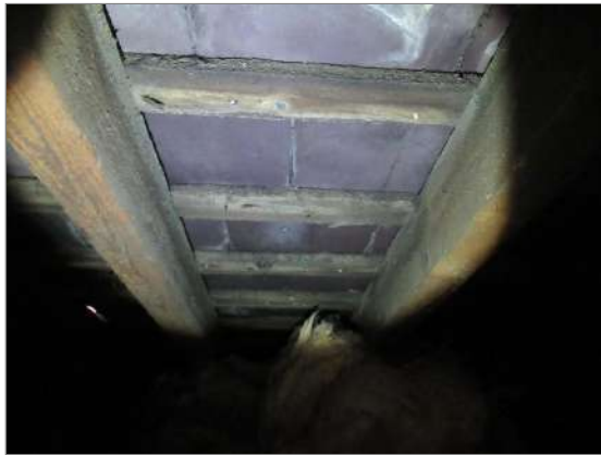
Photo - 62 No sarking present
