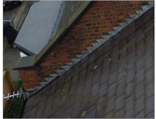
Photo - 15 Damp staining was noted to the front elevation left-hand parapet wall
