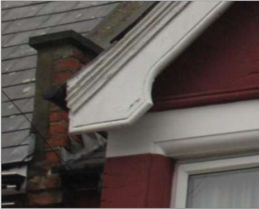
Photo - 61 Weathering was noted to the front elevation soffit and fascia boards
