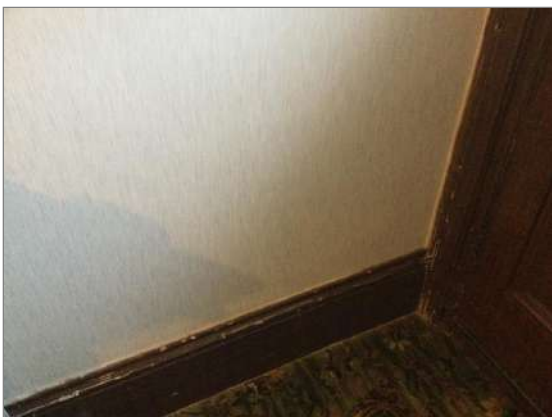
Photo - 85 High moisture meter readings were recorded on the wall adjacent to the front door
