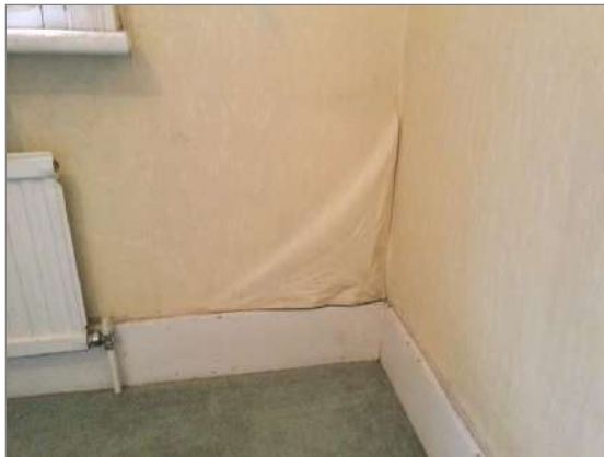
Photo - 93 High moisture meter readings were recorded on the wall in the third left-hand bedroom
