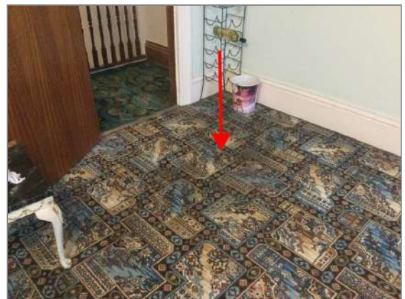
Photo - 100 A dip was noted to the flooring in the front bedroom
