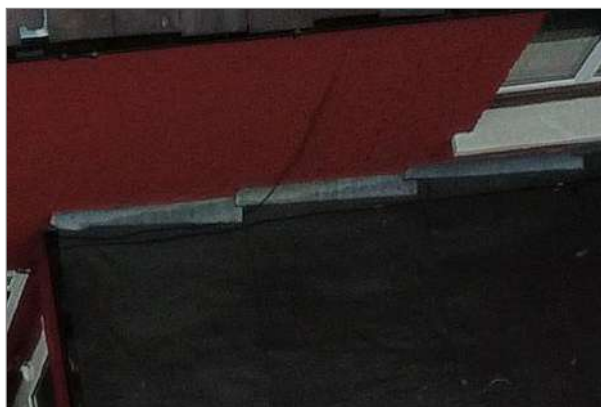
Photo - 21 Gaps were noted to the lead flashing on the flat roof
