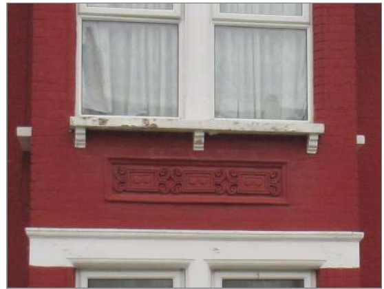
Photo - 44 Weathering was noted to the external concrete window cills on the front elevation
