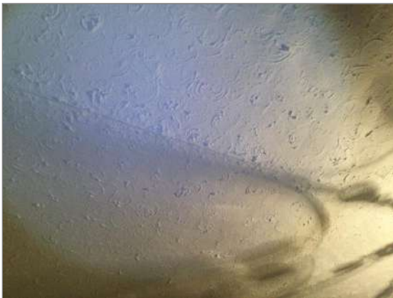
Photo - 73 Cracking was noted to the ceiling in the dining room
