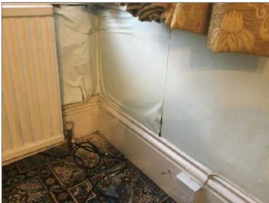
Photo - 89 High moisture meter readings were recorded on the wall in the front bedroom
