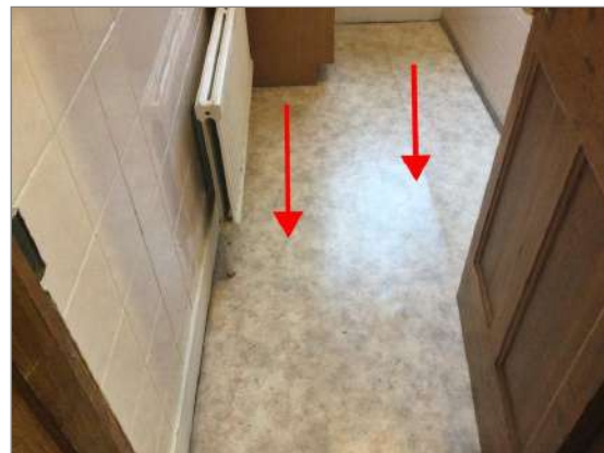
Photo - 104 Floorboards were noted to deflect when traversed in the first floor bathroom
