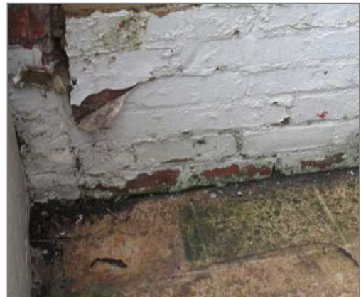
Photo - 143 Damp was noted to the front left-hand boundary wall
