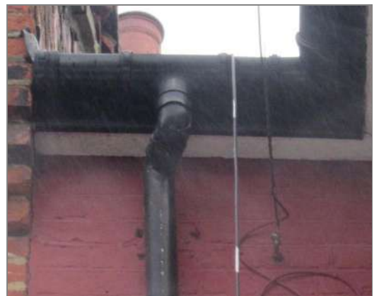
Photo - 24 Staining was noted to the joints of the down pipe on the front elevation
