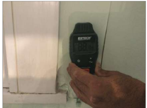
Photo - 88 High moisture meter readings were recorded on the wall in the front bedroom
