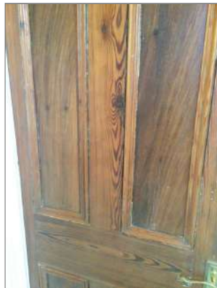
Photo - 117 Shrinkage cracking was noted to the timber door of the third left hand bedroom
