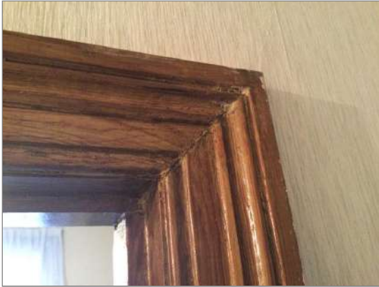
Photo - 115 Example of shrinkage cracking to the timber architrave
