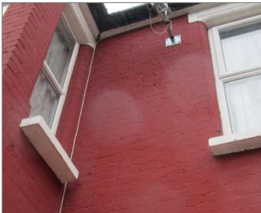
Photo - 31 Gaps were noted in the mortar pointing on the front elevation
