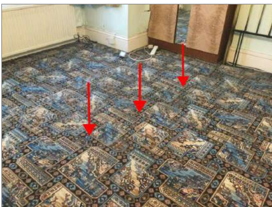
Photo - 101 The flooring was noted to be raised in the front bedroom
