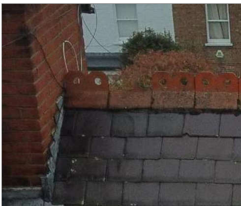
Photo - 12 Broken ridge tiles were noted to the front elevation of the main roof
