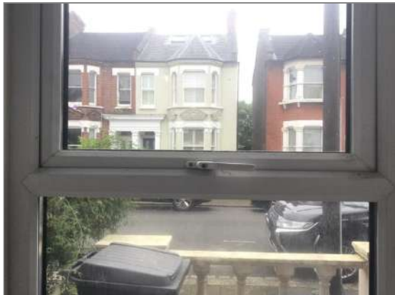
Photo - 41 The window in the front living room was noted to be stiff to operate
