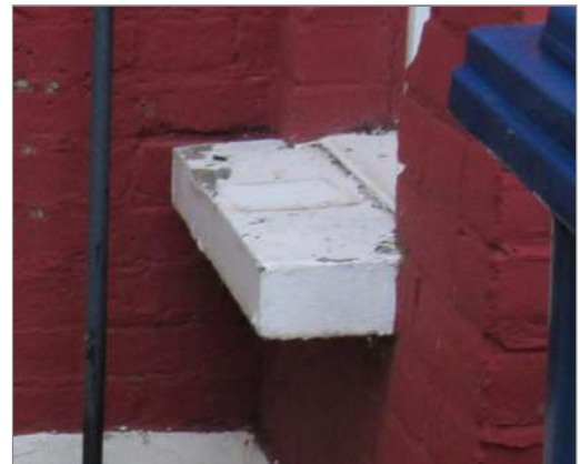
Photo - 46 Weathering was noted to the external concrete window cills on the front elevation
