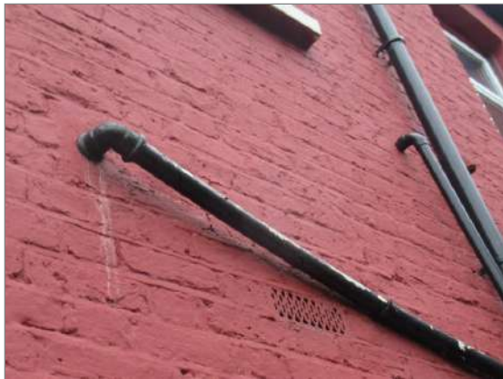
Photo - 25 Staining was noted to the bathroom waste pipe on the rear elevation
