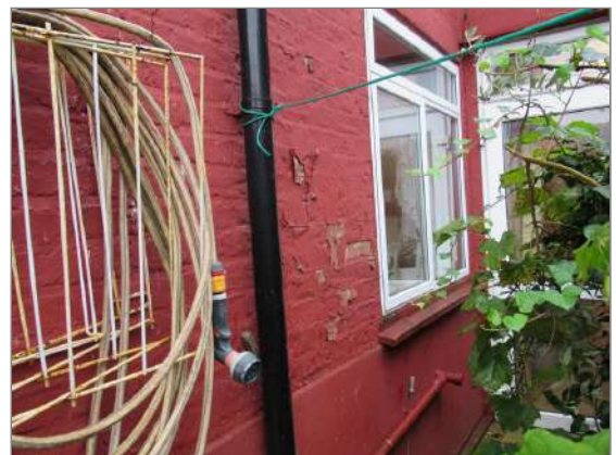
Photo - 40 Damp was noted to the brickwork on the rear elevation
