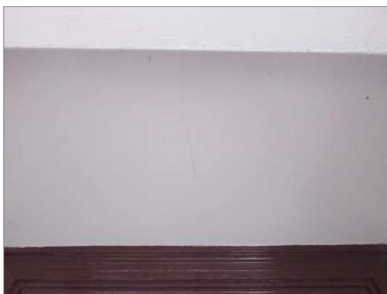
Photo - 56 Cracks were noted to the walls of the porch
