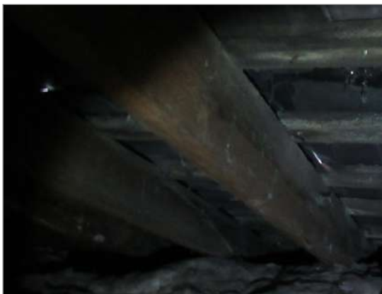
Photo - 66 Gaps were noted to the roof covering
