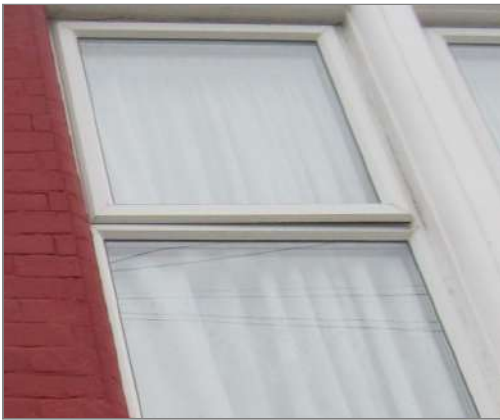
Photo - 43 The window in the front bedroom was noted to be defective and would not close sufficiently
