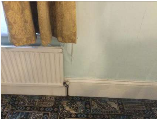
Photo - 87 High moisture meter readings were recorded on the wall in the front bedroom
