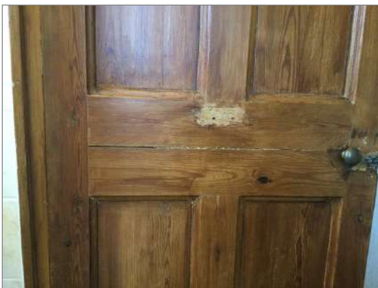
Photo - 119 Shrinkage cracking was noted to the first floor WC timber door
