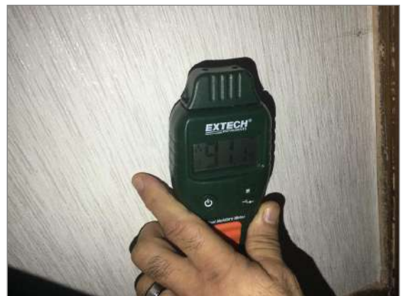
Photo - 86 High moisture meter readings were recorded on the wall adjacent to the front door
