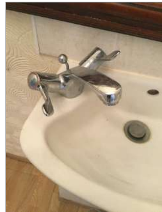
Photo - 121 The tap on the rear left shower room sink was noted to be loose
