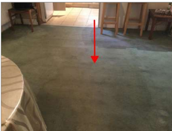
Photo - 99 The flooring was noted to be raised in the dining room
