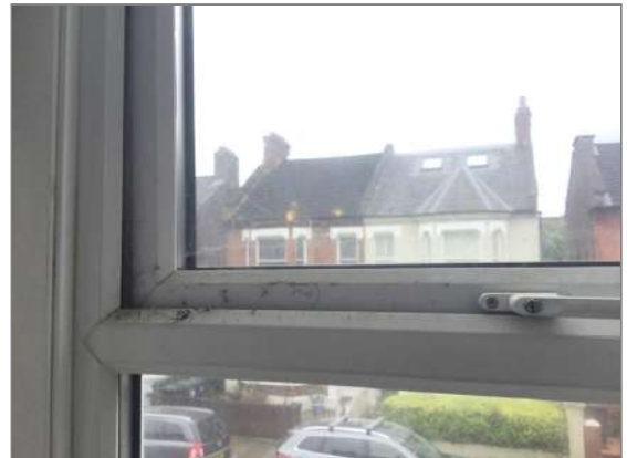
Photo - 42 The window in the front bedroom was noted to be defective and would not close sufficiently
