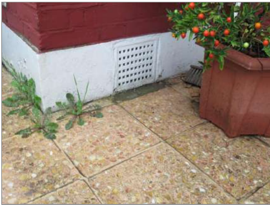
Photo - 35 Damp was noted at the base of the walls on the front elevation
