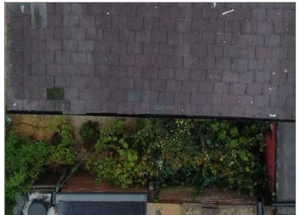
Photo - 26 Slipped tiles were blocking the guttering on the rear elevation
