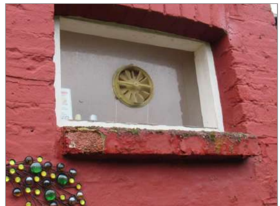
Photo - 48 Damp was noted to the brick window cill on the rear elevation
