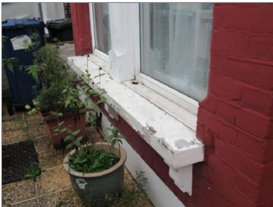
Photo - 45 Weathering was noted to the external concrete window cills on the front elevation
