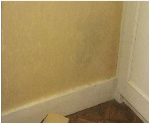
Photo - 83 Damp was noted to the wall in the second left-hand bedroom
