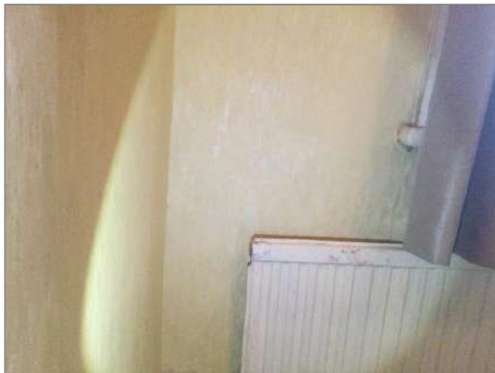
Photo - 95 High moisture meter readings were recorded on the wall in the third left-hand bedroom
