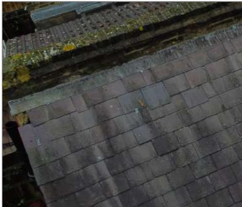
Photo - 16 Gaps were noted between the tiles on the rear elevation main roof
