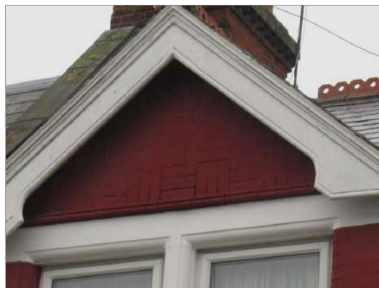
Photo - 60 Weathering was noted to the front elevation soffit and fascia boards
