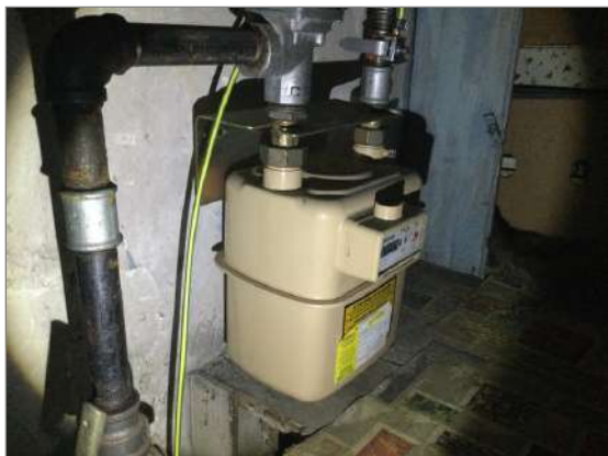
Photo - 129 Gas meter
