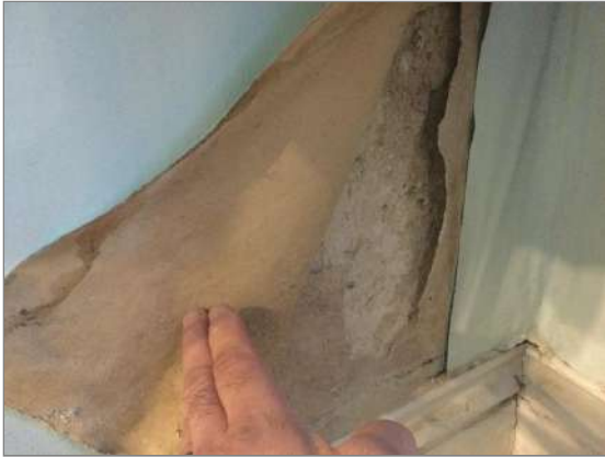
Photo - 81 Damp was noted to the walls in the front bedroom
