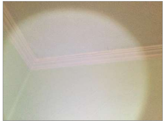
Photo - 78 Hairline cracking was noted to the coving in the first left hand bedroom
