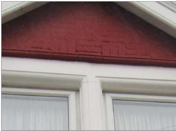
Photo - 29 Gaps were noted in the mortar pointing on the front elevation
