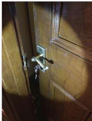
Photo - 113 The second living room door does not engage with latch when closed
