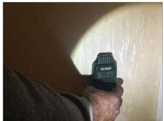
Photo - 92 High moisture meter readings were recorded on the wall in the second left-hand bedroom
