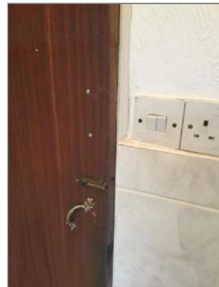
Photo - 114 The rear shower room door does not shut and scuffs the frame when operated
