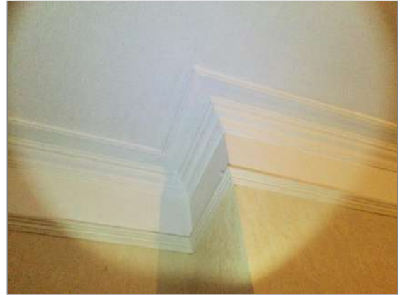
Photo - 72 Hairline cracking was noted to the coving in the second living room
