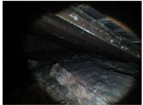
Photo - 63 Damp and mould was noted to the timber roof structure
