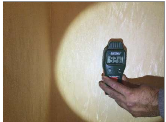
Photo - 96 High moisture meter readings were recorded on the wall in the third left-hand bedroom
