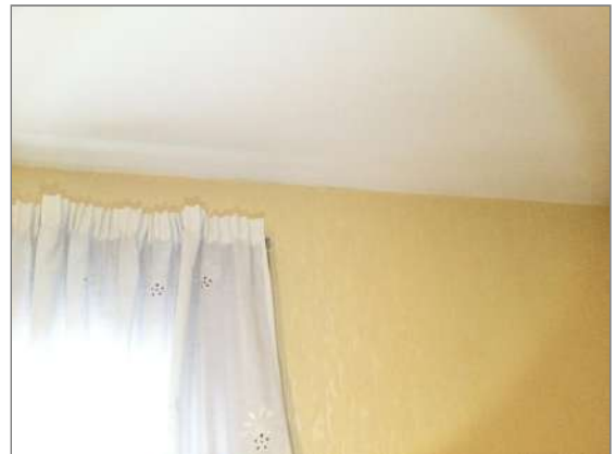
Photo - 80 Perimeter cracking was noted to the ceiling in the second left hand bedroom
