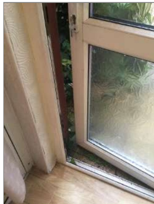
Photo - 53 The rear side door was noted to be defective when operated
