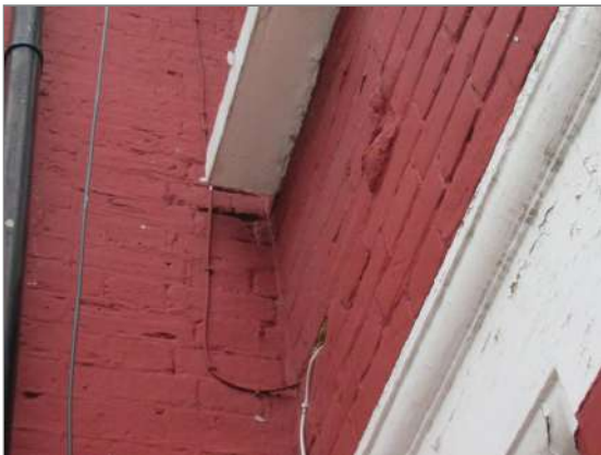
Photo - 37 Damp was noted to the brickwork on the front elevation
