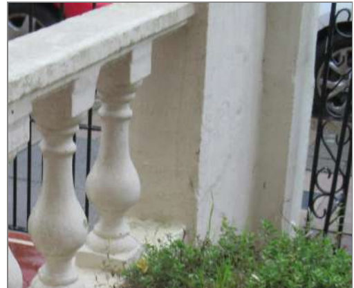
Photo - 139 Cracks were noted to the front right-hand boundary wall
