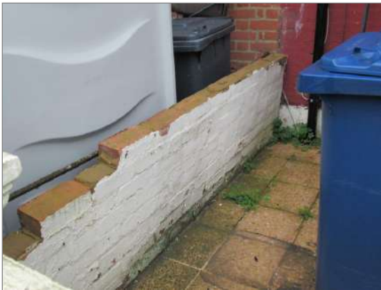
Photo - 142 The front left-hand boundary wall was noted to be leaning and defective
