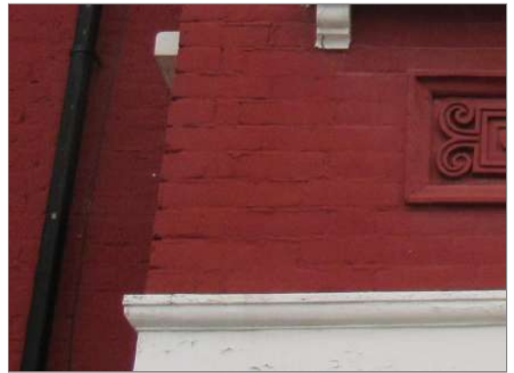
Photo - 30 Gaps were noted in the mortar pointing on the front elevation
