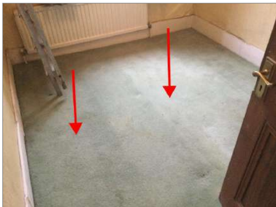
Photo - 103 Floorboards were noted to deflect when traversed in the third left hand bedroom
