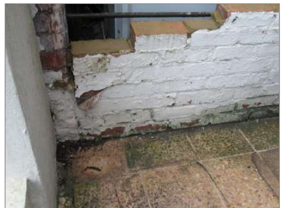
Photo - 141 The front left-hand boundary wall was noted to be leaning and defective
