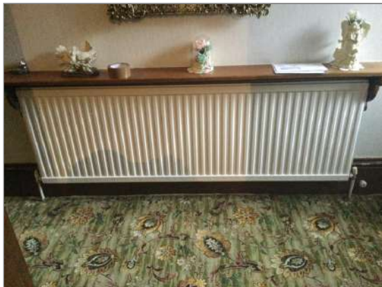
Photo - 133 Radiators throughout
