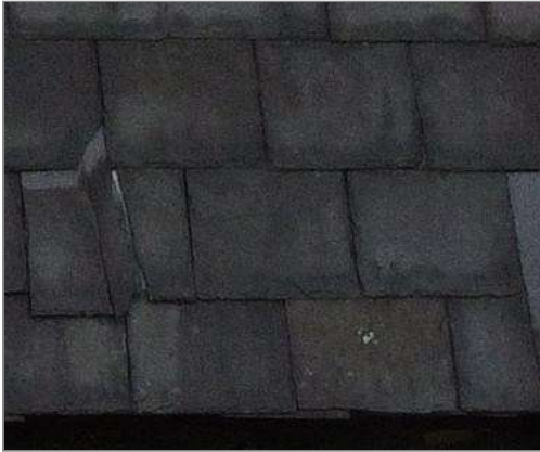
Photo - 14 A broken tile was noted to the front elevation of the main roof
