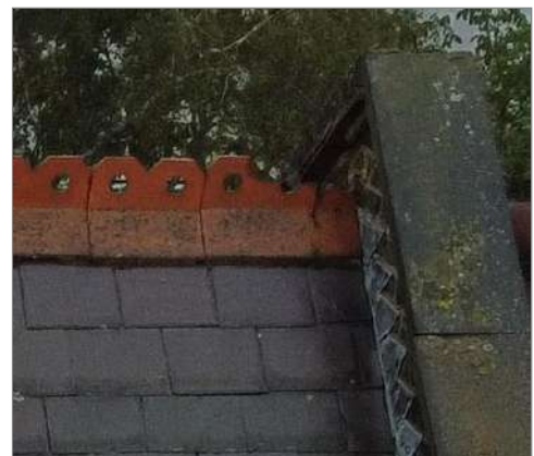
Photo - 13 Broken ridge tiles were noted to the front elevation of the main roof
